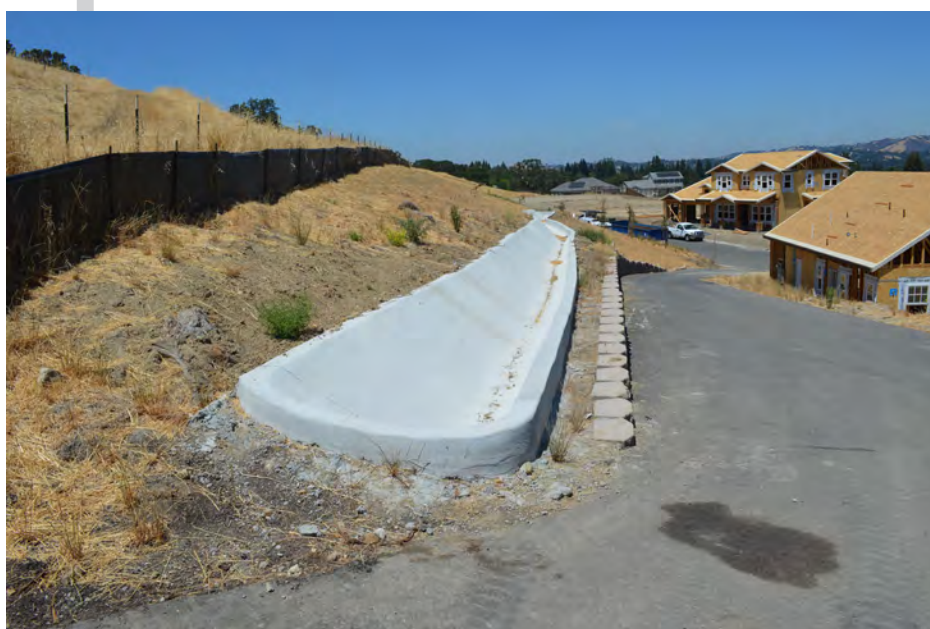
The GHAD has full responsibility for the concrete v-ditch used to collect storm drainage.
